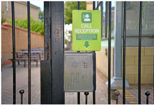
Security gate and intercom/buzzer.
