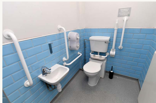
Fully accessible gender neutral toilet in the lobby on the ground floor.
